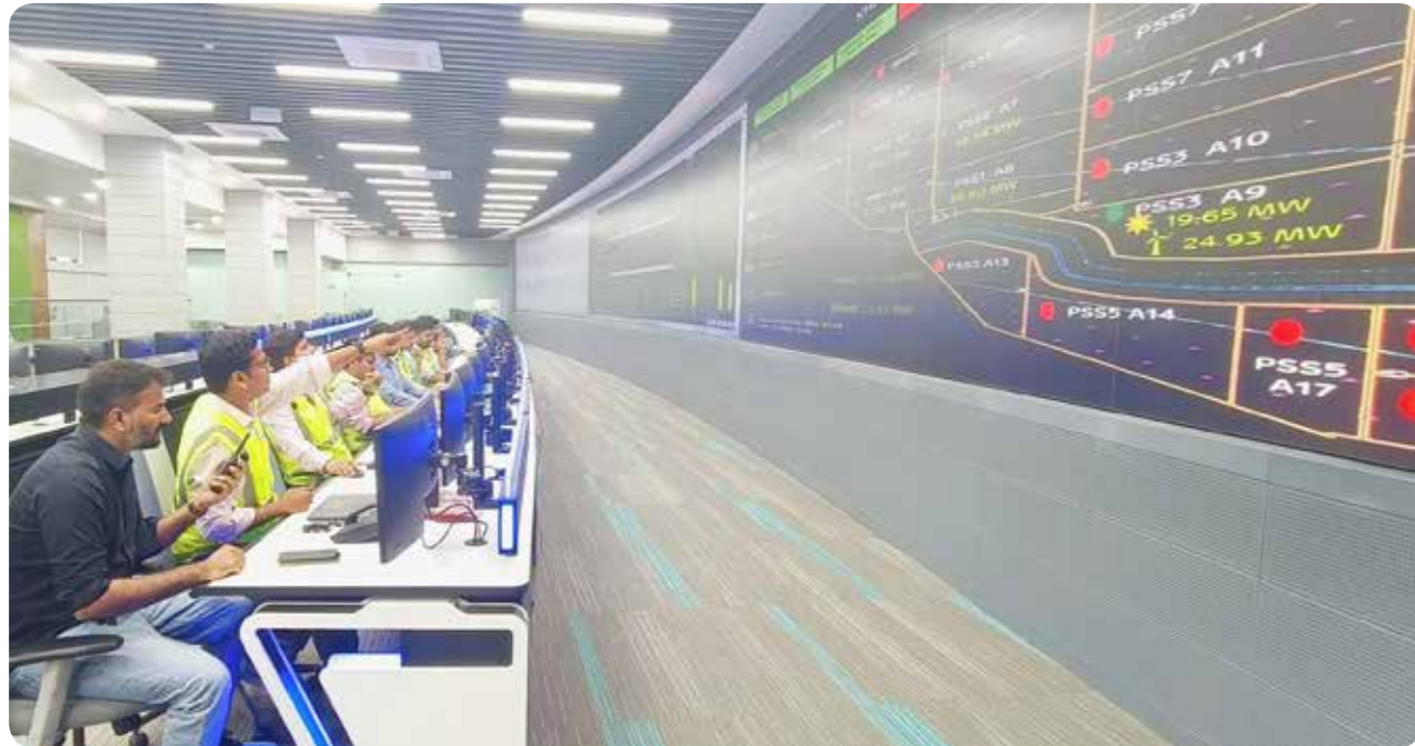
Central Control Room (CCR) at Khavda, Gujarat
